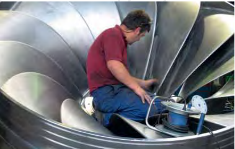
Being aware of the importance of the welding, each Francis runner is consciously assembled by qualified personnel.
